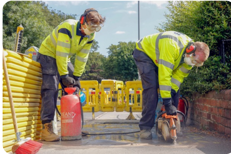
NGN engineers on site undertaking an element of our gas mains replacement work
