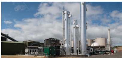
A biomethane production plant
